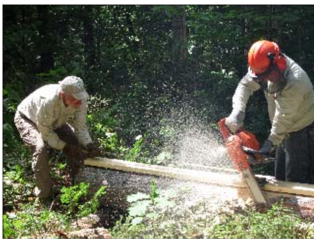
Lester Kenway and Ron Dobra milling a Leeman Brook Lean-to foundation replacement
